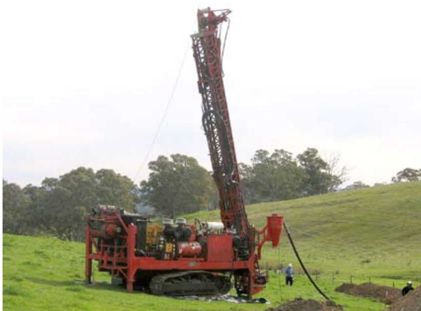
Figure 1 Rig on site for the new drilling program, Bird in Hand, South Australia..
