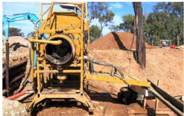
Figure 1 Alluvial plant in operation - May 2007.
