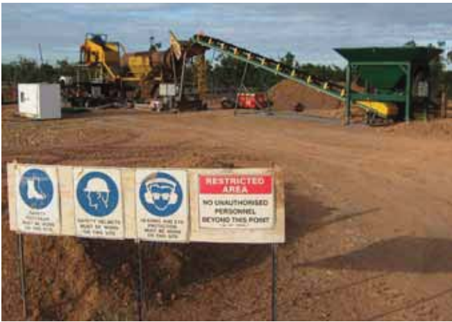
Figure 3 Plant in operation at Sellheim Gold Project, April 2010.
